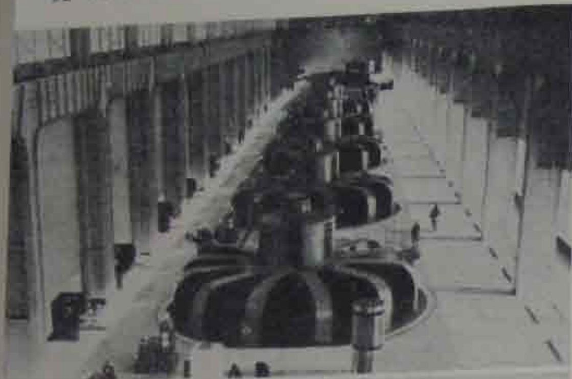
1: Interior of the giant power station at Dnieprostroy. The calmness, cleanness, and order of the neotechnic environment. The same qualities prevail in the power station or the factory as in the kitchen or the bathroom of the individual dwelling. In any one of these places one could "eat off the floor." Contrast with the paleotechnic environment.
